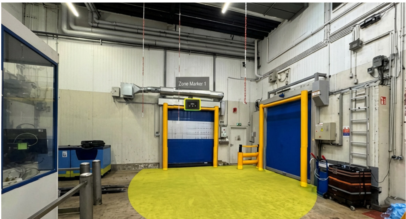
Collision prevention system in Duisburg
